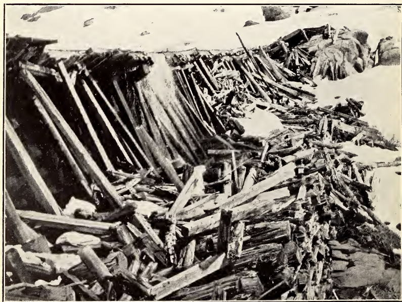
FIG. 2.—SAME, SHOWING DÉBRIS GATHERED AT FOOT OF DAM.
